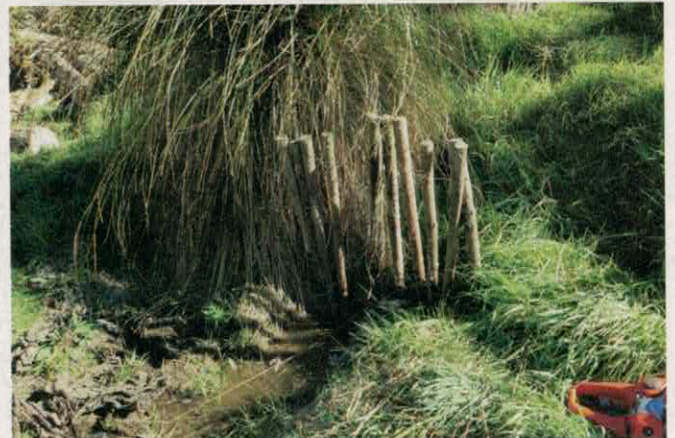
A leaky weir in construction. The posts were placed on an erosion channel in the upper wetland and made ready for branches to be weaved through.
